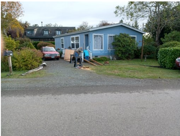
When an elderly parishioner required the use of a wheelchair due to a serious injury to her hip requiring surgery, Brothers Bill Phillips and Frank Roeder (right kneeling) built a ramp with materials donated by the Council
