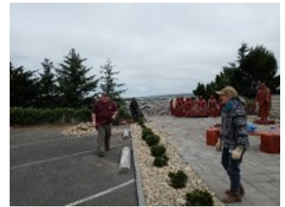
Brother Dan and wife Tammie building a cross walk to the rectory and clearing the gravel
