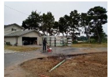
Council Chaplain and Pastor Father Anthony cutting the pavement to prepare for laying the underground electrical
